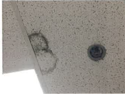
#14: Rm 1409 water stain possible visible mold.
