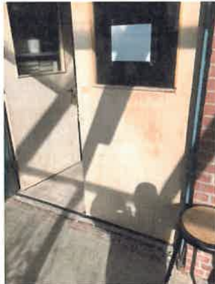
#8: Doors to storage area and greenhouse. Needs a door sweep.
