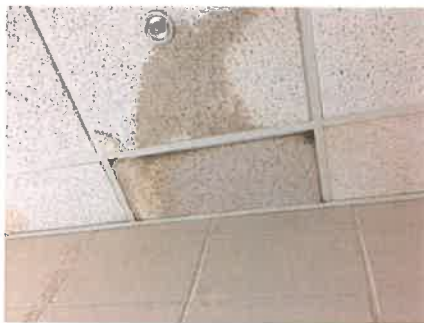
#12: Rm 2207 30% wet ceiling tile; no windows; ceiling vents not operating.
