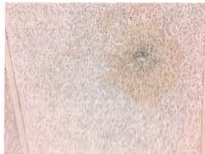
#19: Ceiling next to water main 1700.
