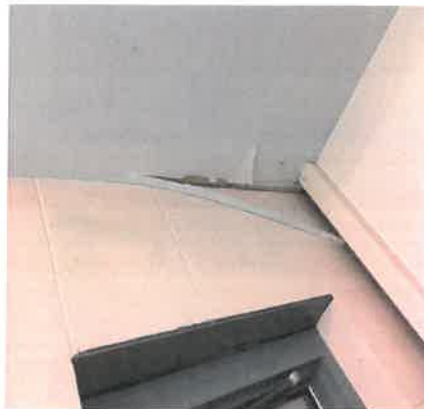
#1: Rm 1506 ceiling/pipe burst two years ago.
