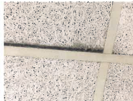
#23: Ceiling in hallway outside gymnasium-possible visible mold.
