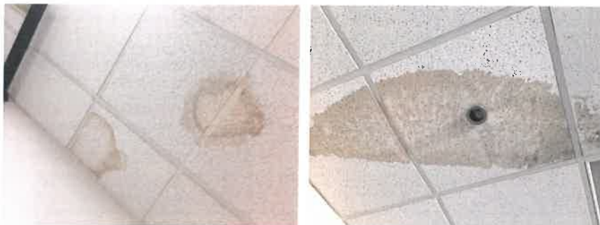
#6: Rm 1515 ceiling stains and floor drain (possible methane gas release).
