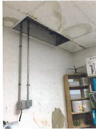
#15: Laundry room. AC on roof may be flooding. Check drip pan.
