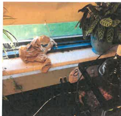
#2: Rm 1506 possible visible mold and moisture.
