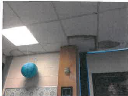
#5: Rm 1515 evidence of roof leak possible mold.
