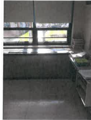
#17: Rm 1203 issues with moisture in the slab.
