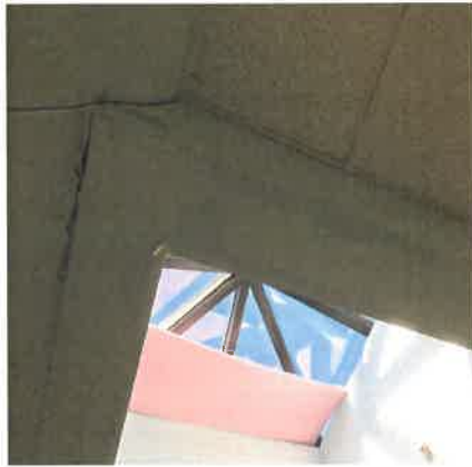
#3: Renovation on water damaged skylight. No barriers erected.
