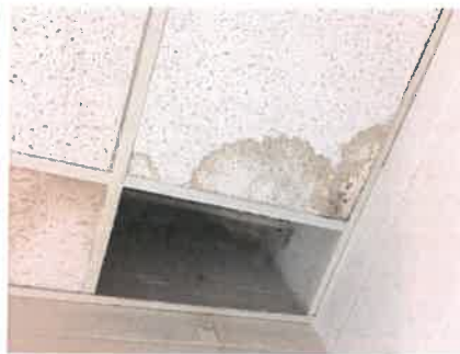
#13: Rm 2210 9% wet ceiling tile.
